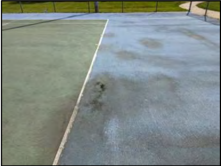
Photo #14 - Settled area at south base line
