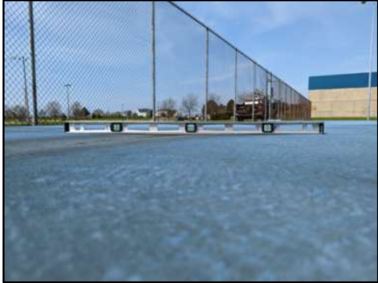
Photo #13 – 1/2" gap under level
