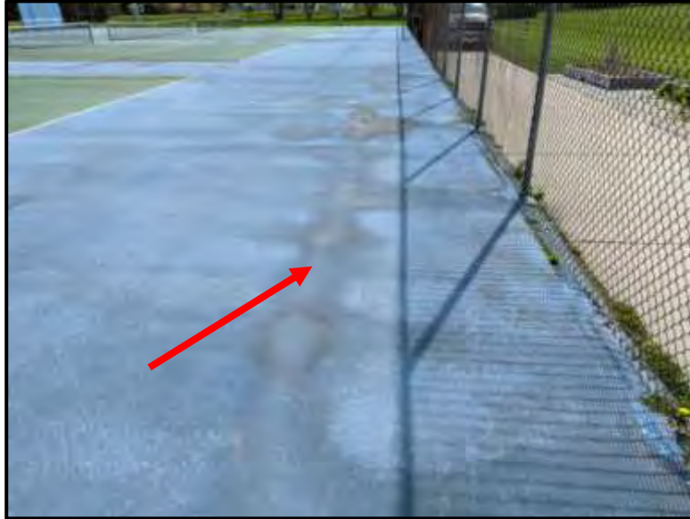
Photo #1 – Settled area over old paving joint
