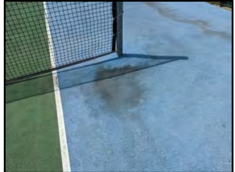
Photo #24 – Settled area at net post footing
