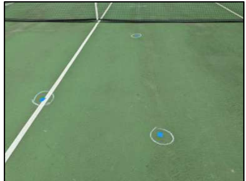
Photo #4 – Low areas over crack below
