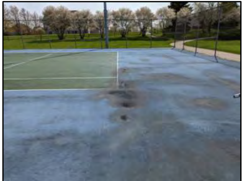
Photo #12 – Settled area over paving joint
