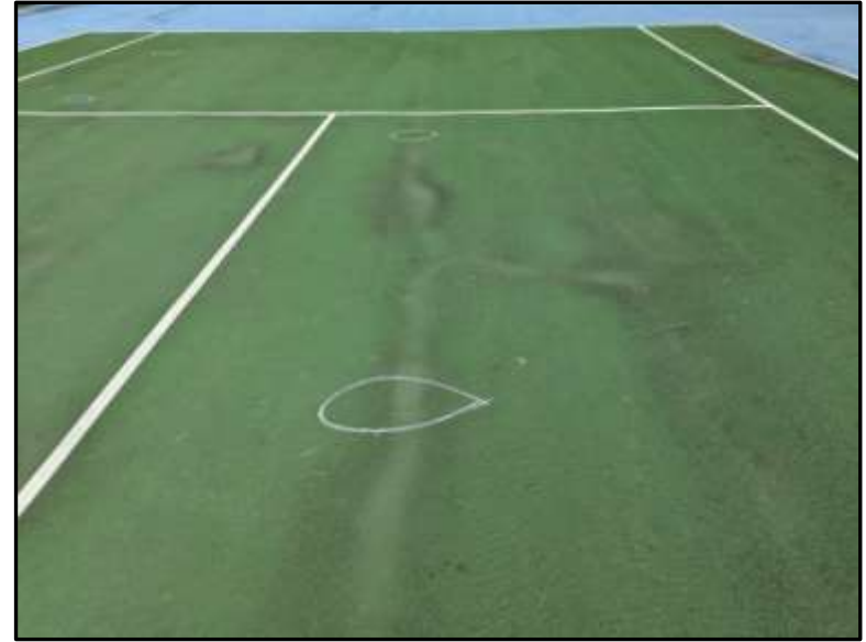
Photo #22 – Settled area over crack
